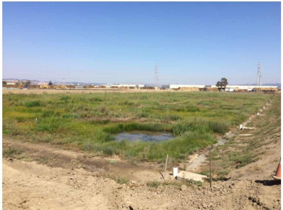
Figure 4.7 Oro Loma Horizontal Levee in the Construction Phase. Photo Credit: Oro Loma Sanitary District.
