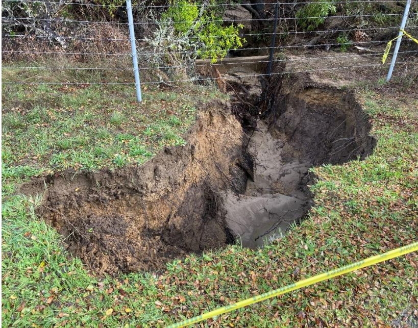
Canada Road – Culvert/Sink Hole
