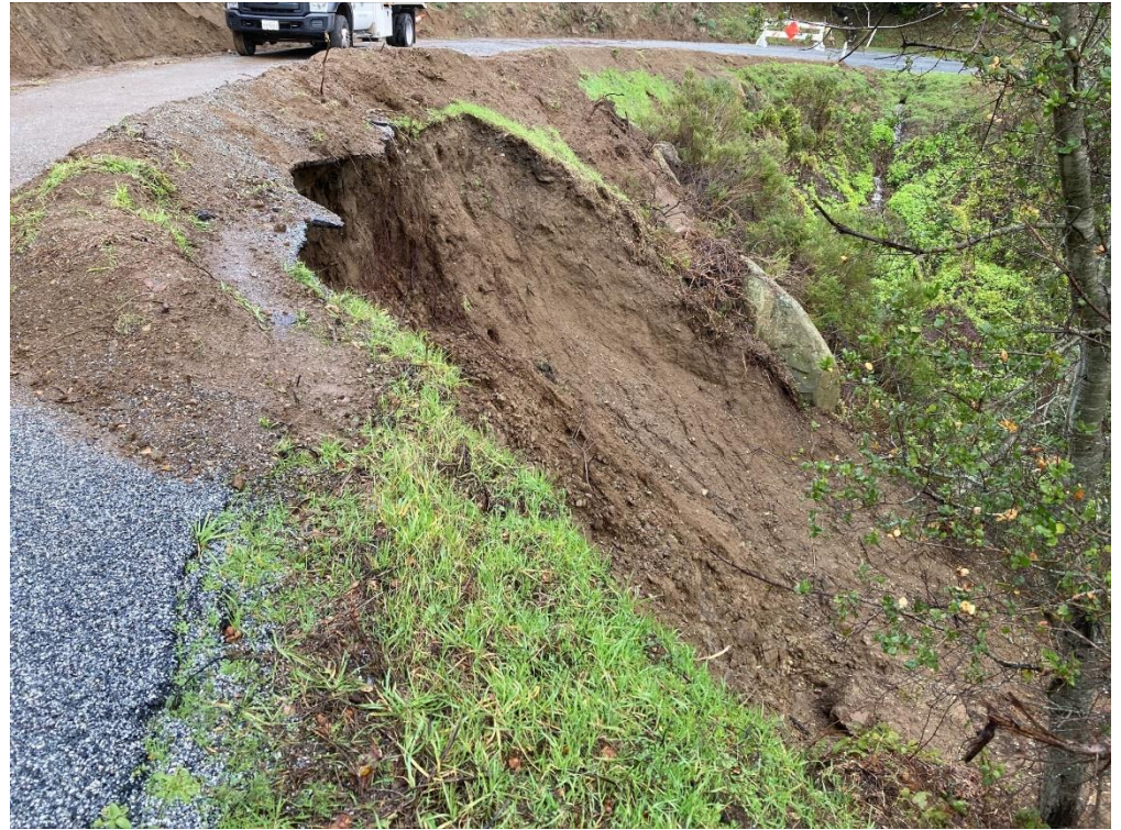
Old La Honda Road – Roadway Closed
