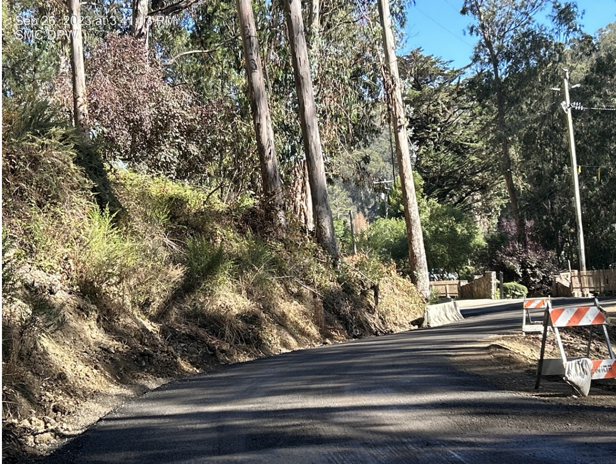
2180 Higgins Canyon Road – Slipout and Earth Movement
