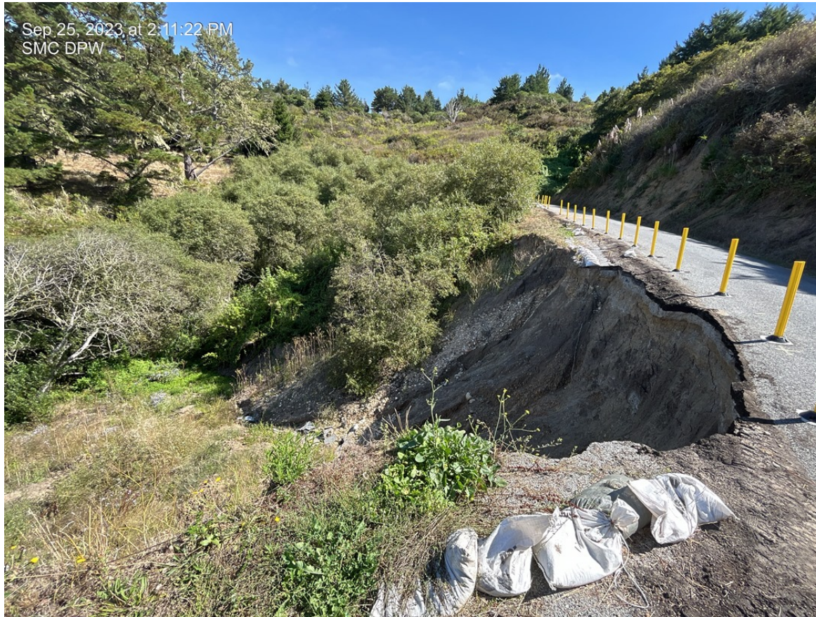
2665 Higgins – Damage from January Storms
