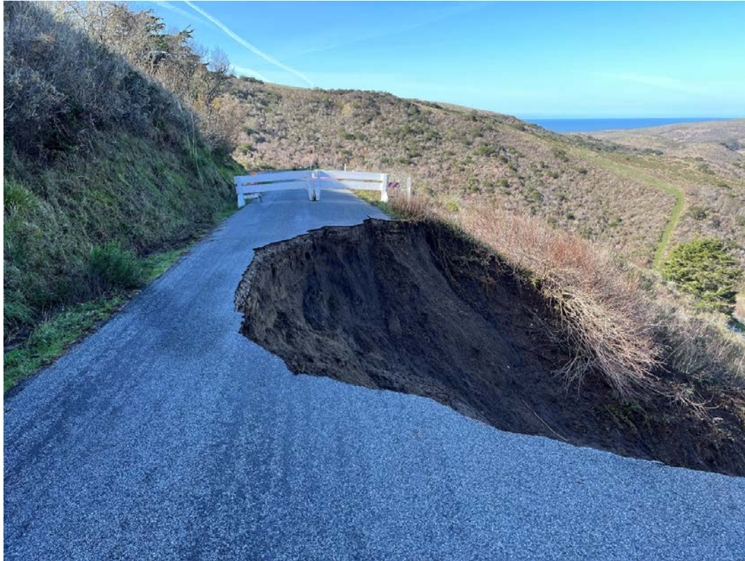
Stage Road #1 – Slide Damage from January Storms
