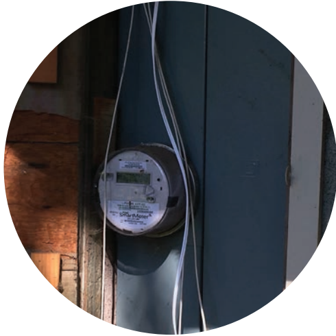
Existing 200-amp main electrical panel
