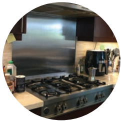
Existing 5-burner 36" gas cooktop
