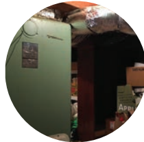
Existing Gravity-fed floor furnace
