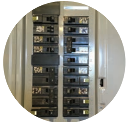
Existing 100-amp laundry room subpanel
