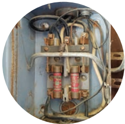
Existing 60-amp main fuse box
