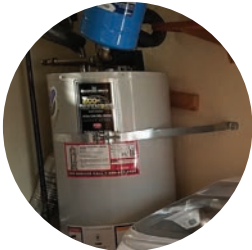
Existing 40-gallon gas water heater
