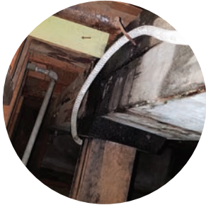
Existing Floor, no insulation
