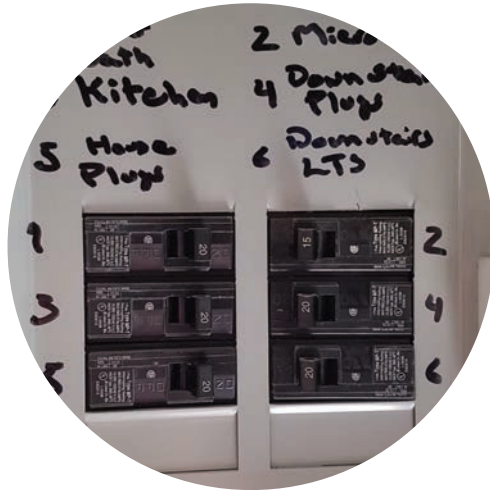
Existing 60-amp electrical subpanel
