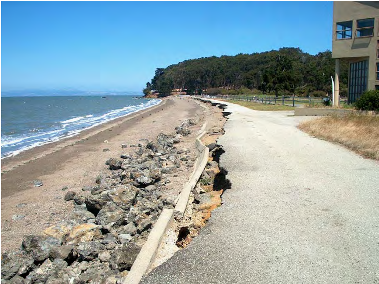
Figure 5-1: Erosion along the Eastern Promenade trail.
