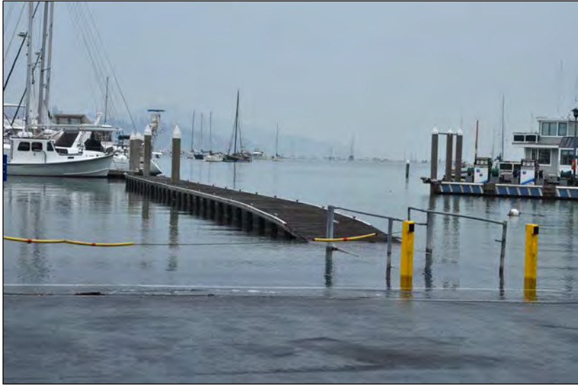
Figure 5-3: Flooding around float abutment due to king tide, CCC (2019).
