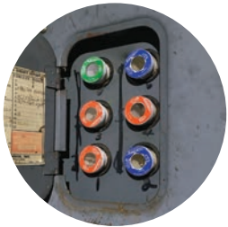
Existing 60-amp subpanel
