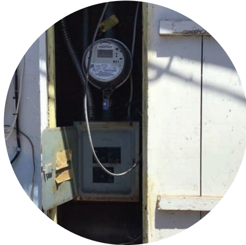
Existing 100-amp main electrical panel
