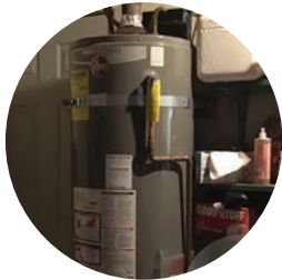
Existing 50-gallon gas water heater
