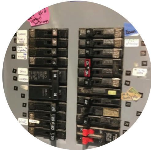
Existing 100-amp subpanel
