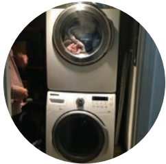
Existing 7.5 cu ft electric resistance dryer
