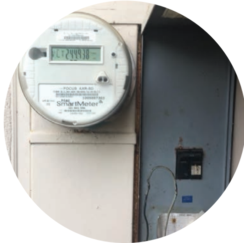
Existing 100-amp main electrical panel
