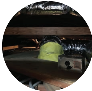
Existing Ductwork, good insulation
