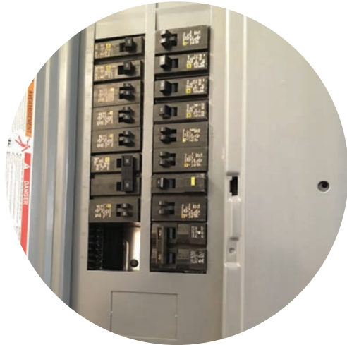
Existing 100-amp subpanel
