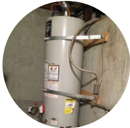
Existing 40-gallon propane gas water heater
