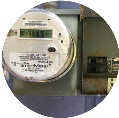
Existing 100-amp main electrical panel
