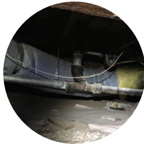
Existing Ductwork, poor condition
