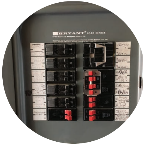
Existing 100-amp subpanel
