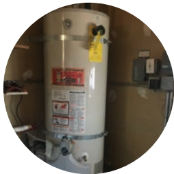
Existing 50-gallon gas water heater
