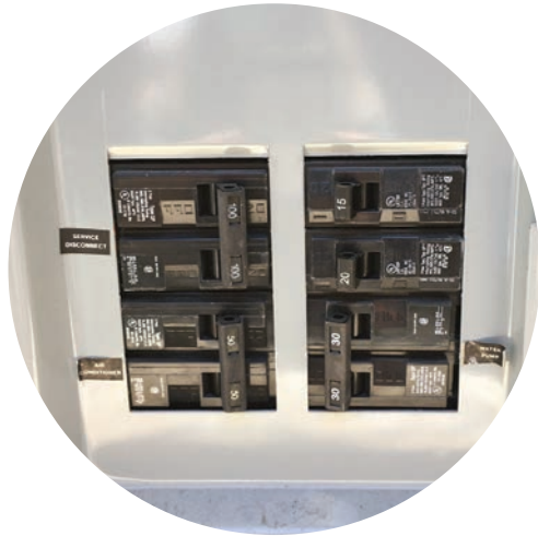
Existing 100-amp main electrical panel
