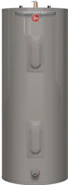
Existing 50-gallon electric resistance water heater
