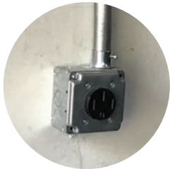
Existing 50A Outlet
