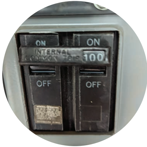
Existing 100-amp main electrical panel
