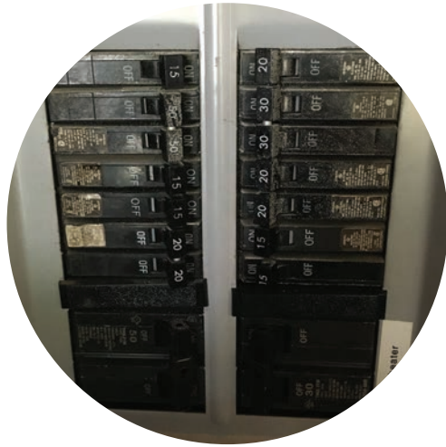
Existing 100-amp subpanel
