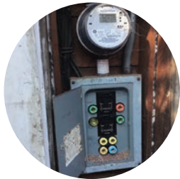
Existing 100-amp fuse box
