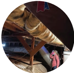
Existing 40-gallon gas water heater
