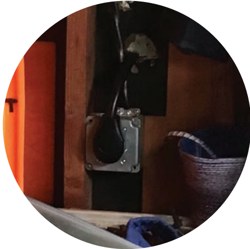
Existing 50A/240V outlet for EV in garage
