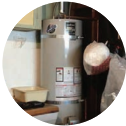
Existing 50-gallon gas water heater
