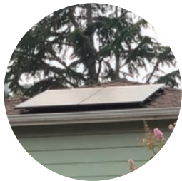
Existing Rooftop solar system
