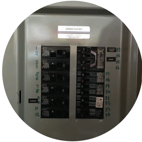
Existing 100-amp subpanel
