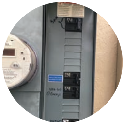
Existing 125-amp main electrical panel
