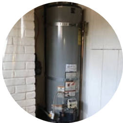
Existing 40-gallon gas water heater
