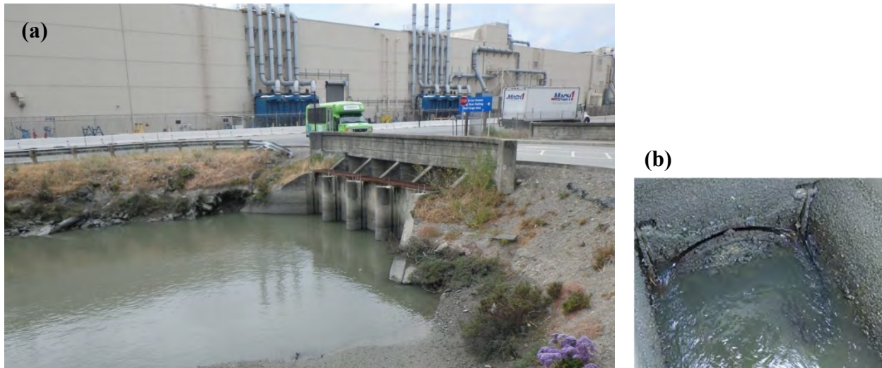
Figure 2-10. San Bruno Channel. (a) Tide gate Structure, Downstream Side (b) Flap Gate
